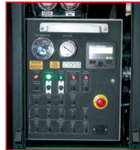
Main Controls with E-Stop
