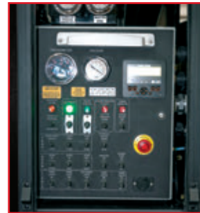
Main Controls with E-Stop
